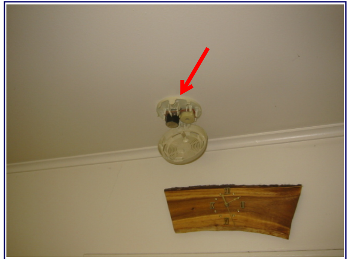
Disabled smoke detector.
