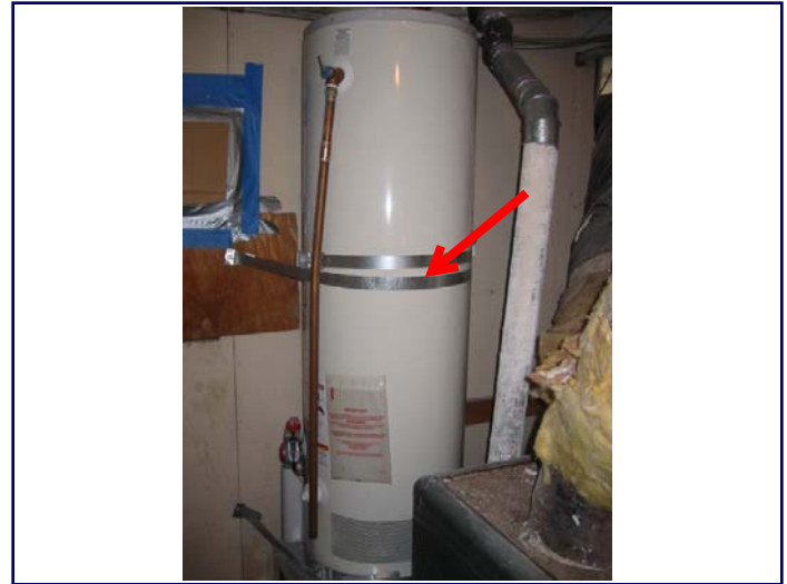
Improperly strapped water heater.
