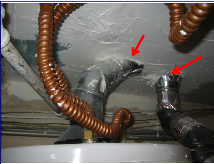
Inadequate clearance to combustable materials and improper flues.
