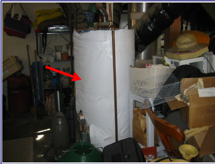
Improperly strapped water heater.
